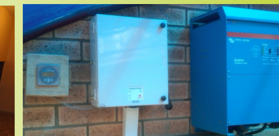
8kW Inverter Backup System in Maitama, Abuja
