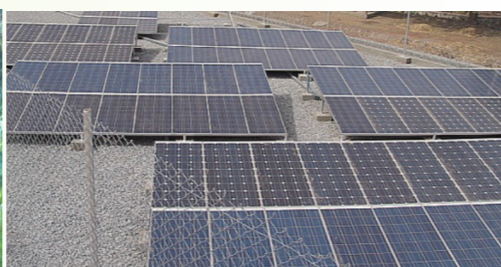
30kW Solar Power System in Minna
