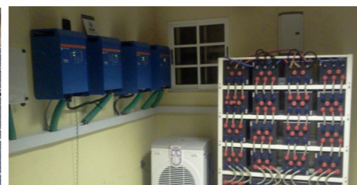
25kW Inverter Power System in Maitama, Abuja
