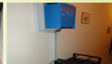
5kW Inverter Backup System in Jabi, Abuja
