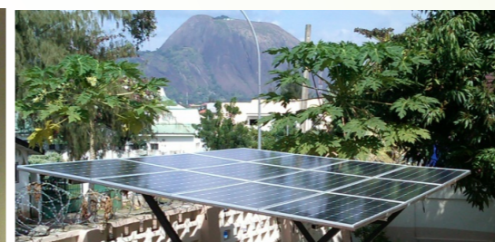
10kW Solar Power Backup System in Wuse 2, Abuja
