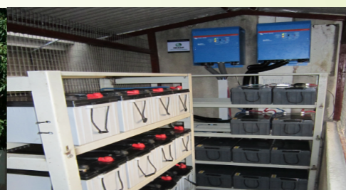
15kW Inverter Backup System in Lekki
