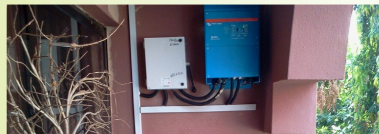
10kW Inverter Power System in Asokoro, Abuja
