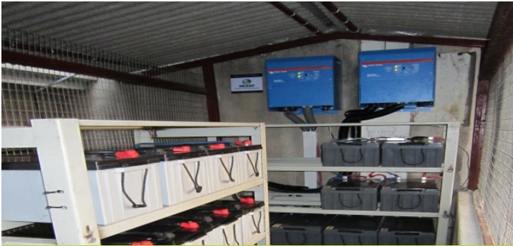
15kW Inverter Backup System in Lekki
