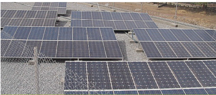
30kW Solar Power System in Minna
