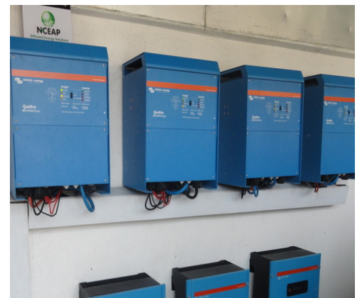
40kW Solar Power System in Lekki, Lagos
