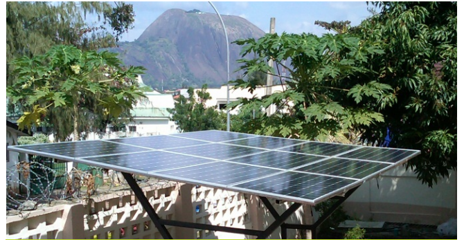
10kW Solar Power Backup System in Wuse 2, Abuja
